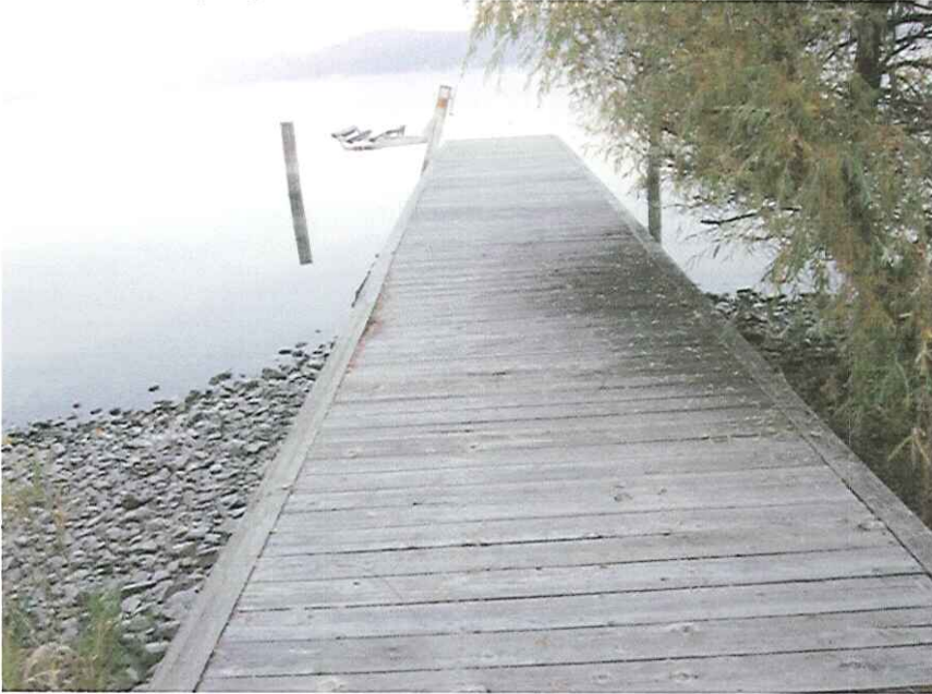
Photo 3: Existing dock at 13 Nerie Road with one boat lift. Note the rotted section on the left of dock (N side) and two old pilings at the end of dock.
