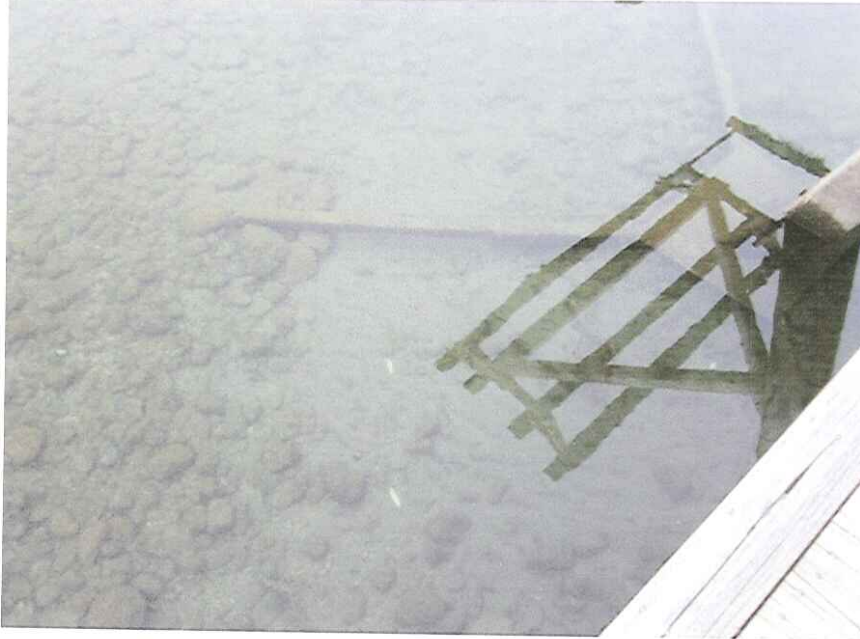
Photograph 7: Substrate under the existing boat lift at 13 Nerie Road – potential boat scour due to the shallow littoral shelf
