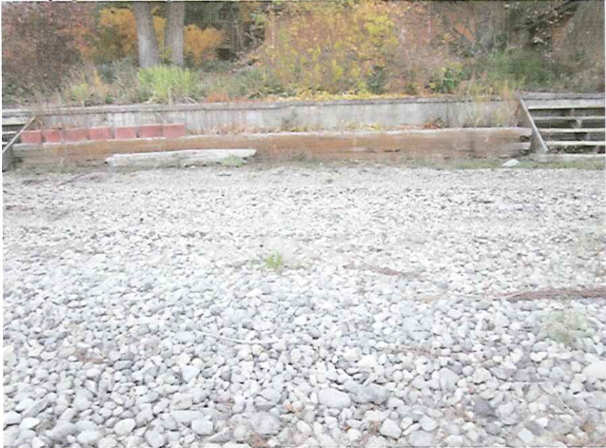
Photograph 1: Existing retaining wall at 13 Nerie Road, Vernon, BC located just above the HWM
