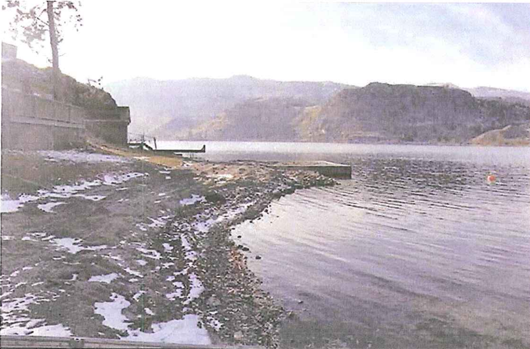
Photo C. View looking west from inside the cove. This area was disturbed recently to place a storm outfall drain from eastside road. This area should be restored and replanted with native grass, shrub and trees. Planting trees along the north shore of the cove has the added benefit of adding shade as well as leaf litter and insect drop to the lake. Insect drop is an important food item for fish.
