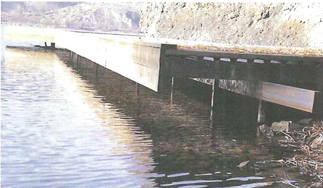
Photo D. View looking west from inside the cove. The lower batter board (2' x 8' skirting) and the lower metal 2' x 5' metal tube support beam both run the length of the dock and are both at high water of 338.0 m geodetic elevation. The board and the beam should be removed to allow for less shading and allow for a more natural wave action. The lower support structure should be 0.6 m above high water or 338.6 m. Currently the top of the deck is approximately 338.6 m.
